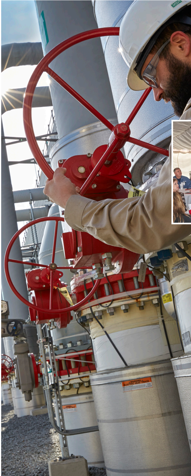
Employees at the Tenaska Westmoreland Generating Station near Smithon, Pennsylvania, regularly monitor equipment to ensure the plant is operating safely and efficiently.
